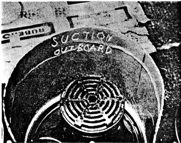
Figure 4. Suction outboard valve.
